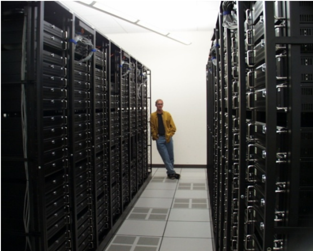
One of the many rows of Linux servers at Google's server farm
